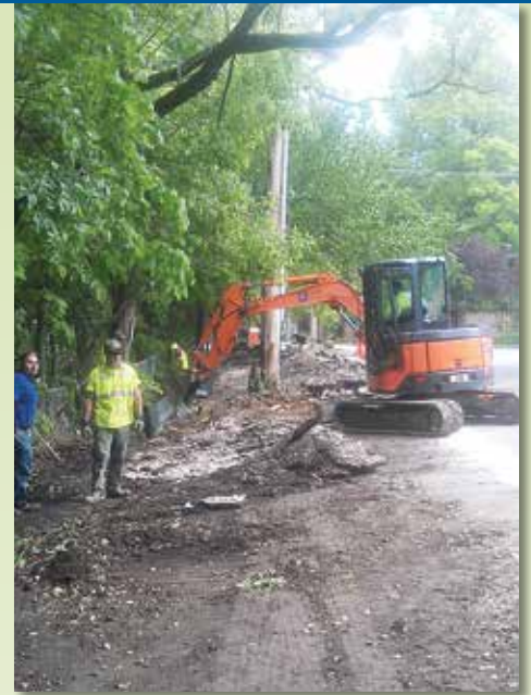
Work crews begin the process of asphalt removal from the Bolton Street Synagogue parking lot.
